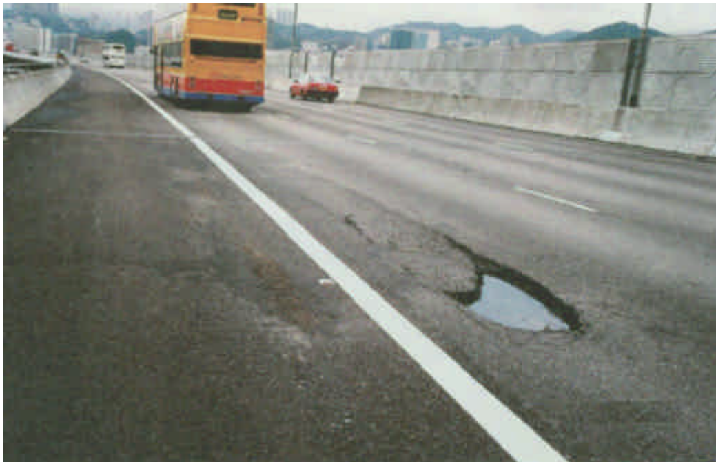
Photograph 2 An example of a defect on the road surface of the West Kowloon Expressway Viaduct (para. 2.5 refers)
