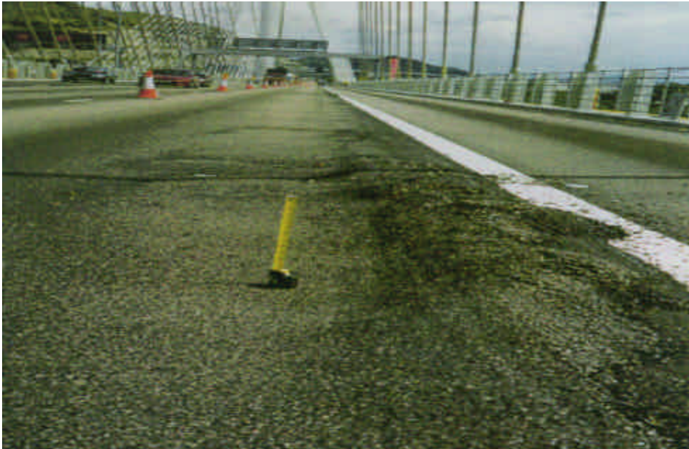
Photograph 1 An example of a defect on the road surface of the Ting Kau Bridge (para. 2.5 refers)
