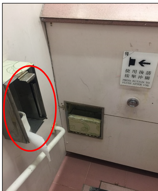
Photograph 4 Defect in toilet paper holder
