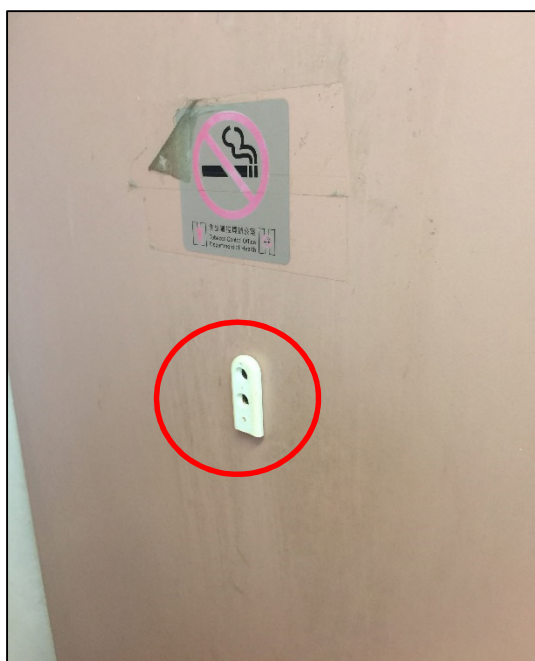
Photograph 3 Defect in coat hook
