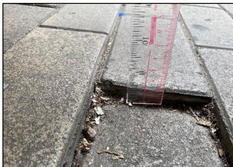
(e) Stepping of paving blocks greater than 10 mm at South Wall Street
