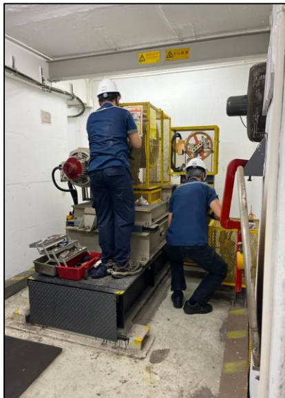
(a) In lift machine room
