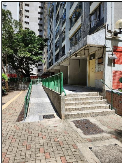
(a) Tactile warning strips not provided and nosing of a staircase not in contrasting color
