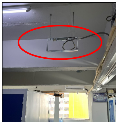
(b) Missing/defective exit signs and/or directional signs
