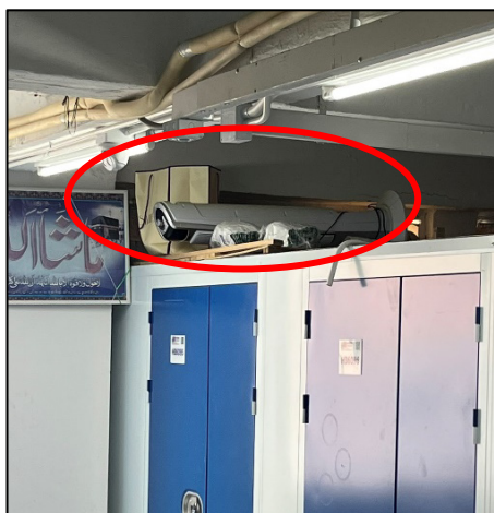
(a) Undesirable arrangement of storage cubicles
